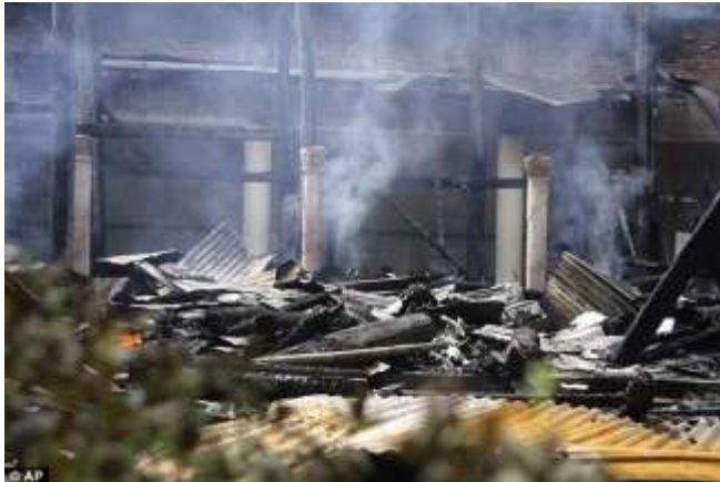
Burning: Smoke rises from the remains of a Buddhist temple that was torched in Ramu. The attacks were sparked by a photograph on Facebook, which Muslims claimed was insulting to Islam
